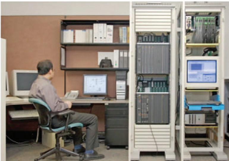
Figure 1. SDS1 Development and Validation Test Rig
