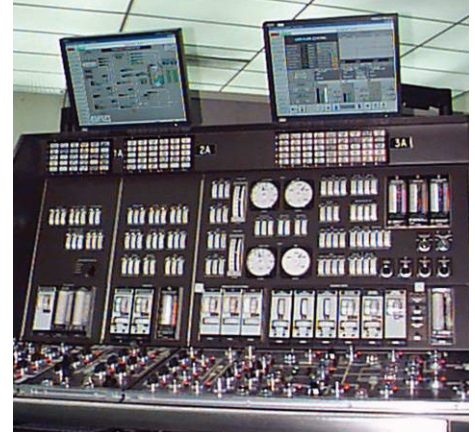
Figure 4: Installed Foxboro I/A Series System on simulator (upper), old feedwater hard panel control (lower)
